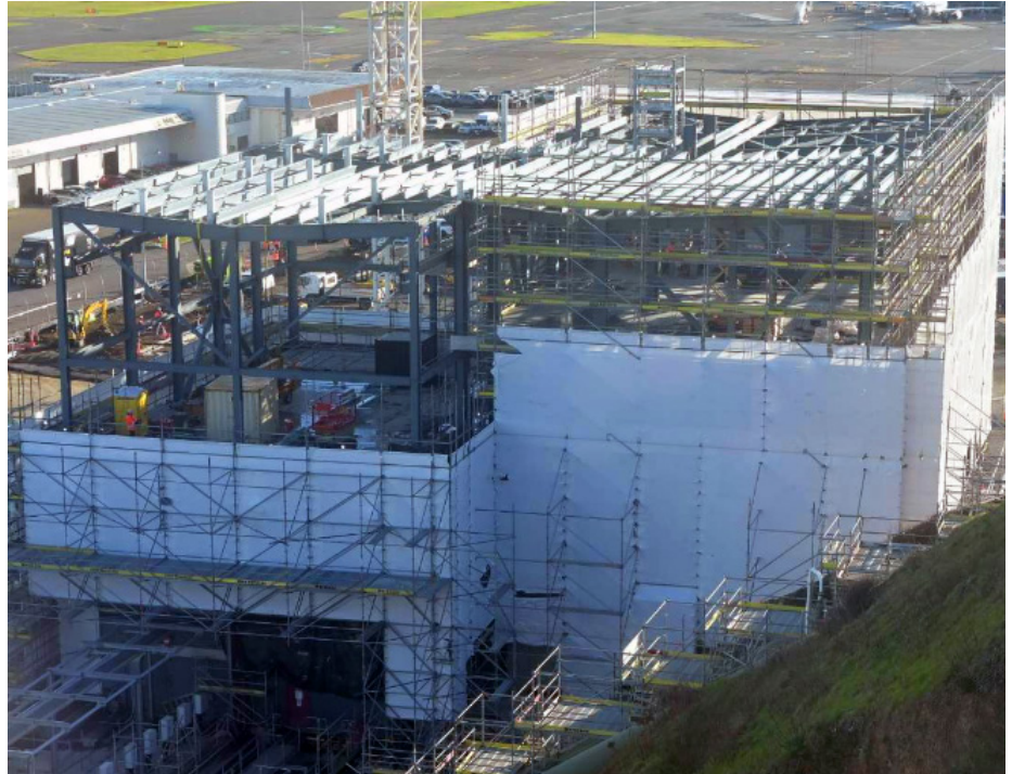
Above: Construction on the Main Process Building continues at pace as the 'purlins' or roof beams are put in place.
